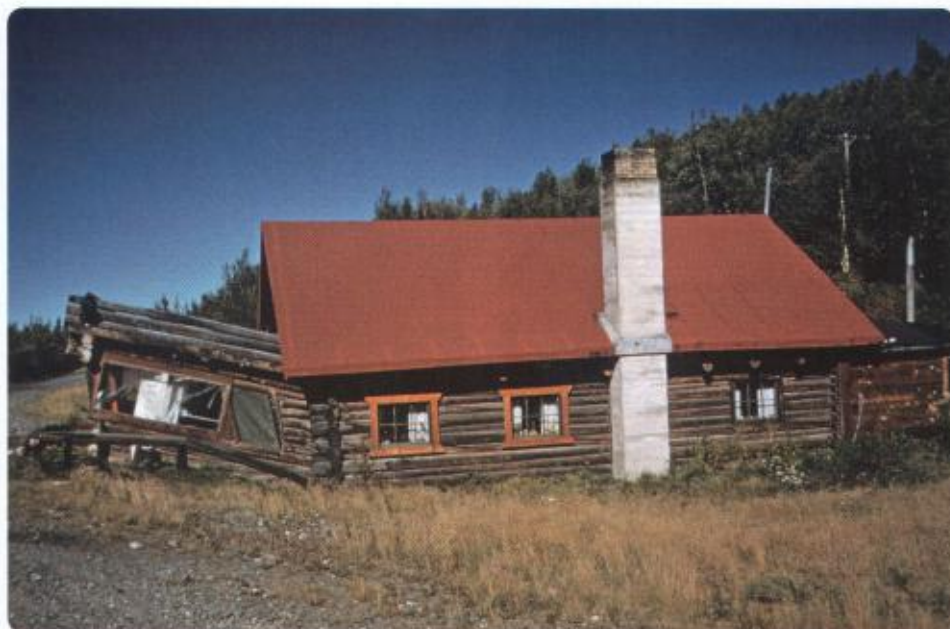
Figure 5 This house was damaged as the permafrost below it thawed.
