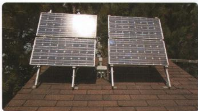
Figure 1 These solar panels change orientation throughout the day to capture the most sunlight.
