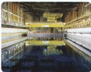
Figure 7 Nuclear waste is stored in temporary facilities.
