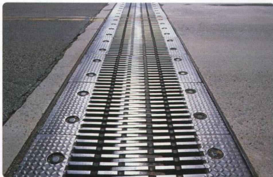
Figure 5 Special expansion joints in this bridge accommodate thermal expansion and contraction when temperatures change, preventing buckling and cracking.
